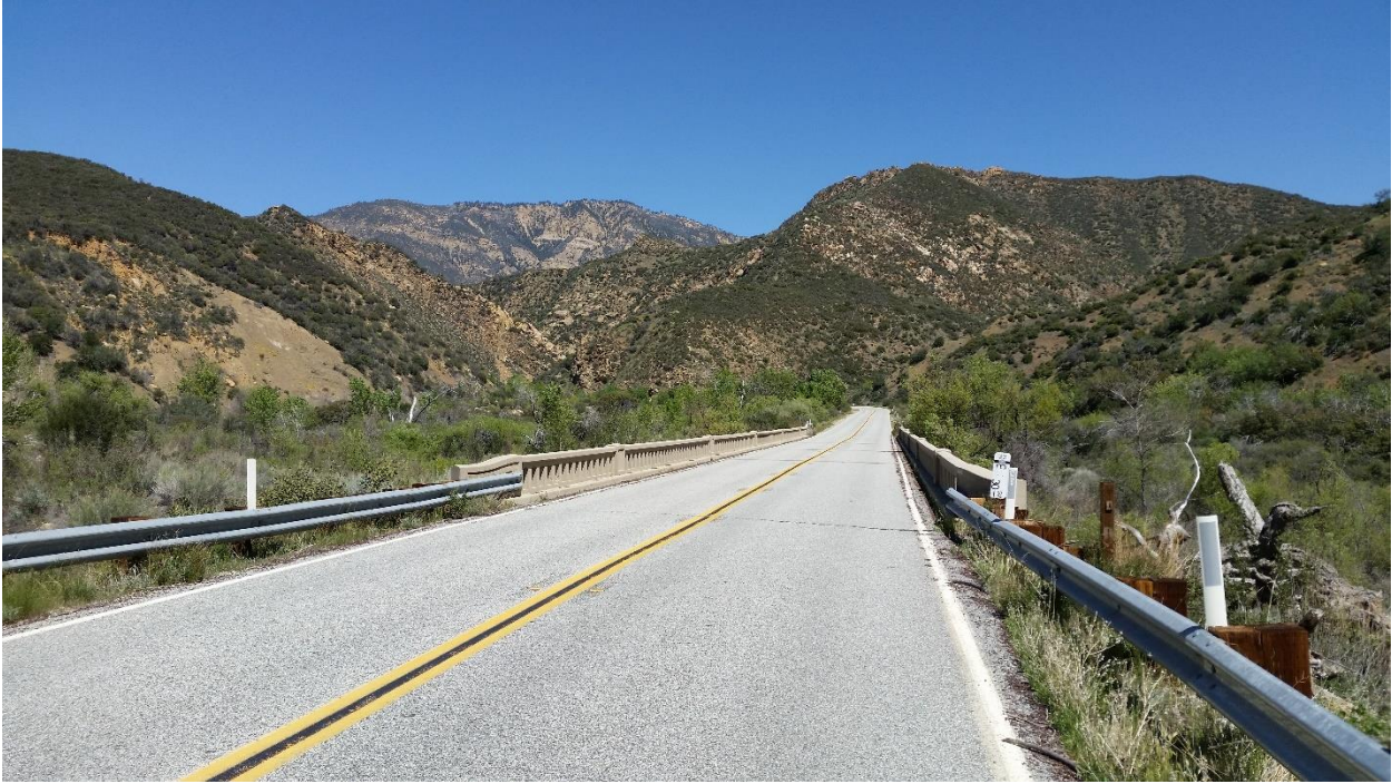
Former US 399 (now State 33) in Sespe Gorge at the 1932 Sespe Creek Bridge (52-0078). Courtesy – Michael F Ballard
